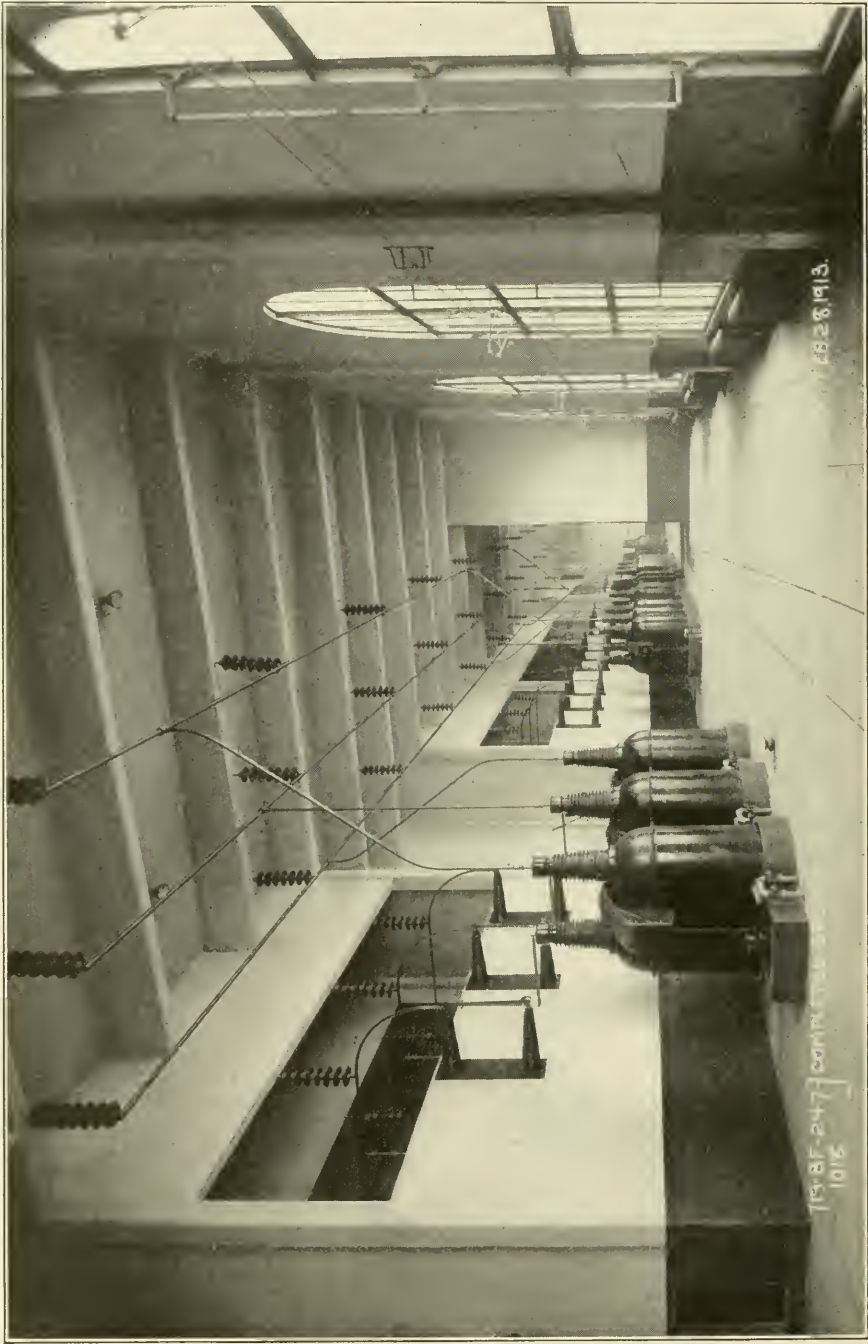
INSTALLATION OF GENERAL ELECTRIC PNEUMATICALLY-OPERATED HIGH TENSION SWITCHES FOR THE MISSISSIPPI RIVER POWER COMPANY
